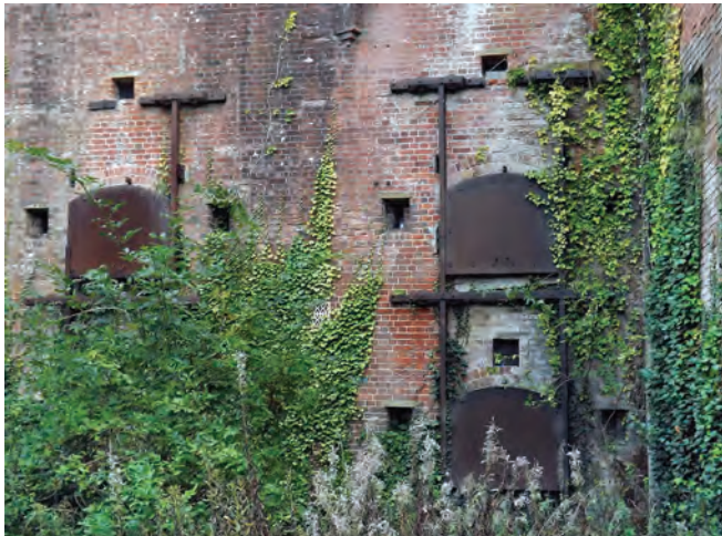
Metal shutters still in position at Fort Purbrook. These would have been lowered during an attack on the fort to enable the larger guns to fire down the length of the moat
